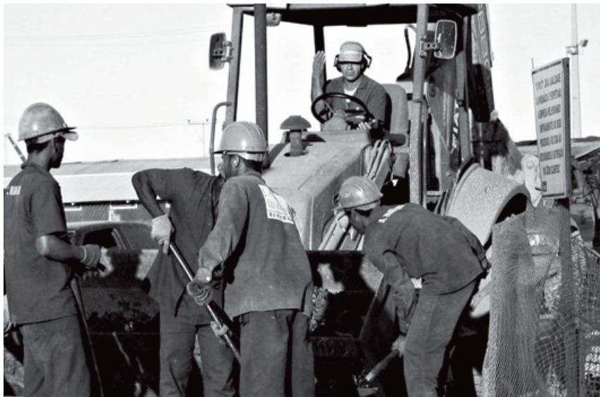
More than 9 000 people have worked on the construction of the Veracel Pulp Mill in Brazil, which will start operating in mid-2005.
